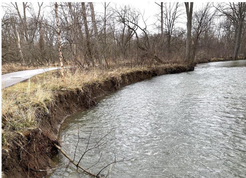
Severely eroded banks in Phase 2 segment
